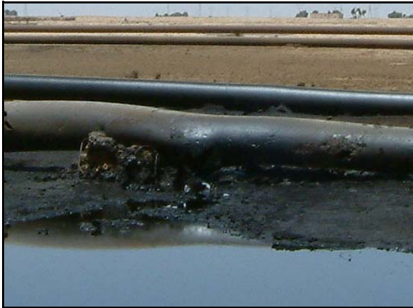
Broken Pipe During Project RIO
